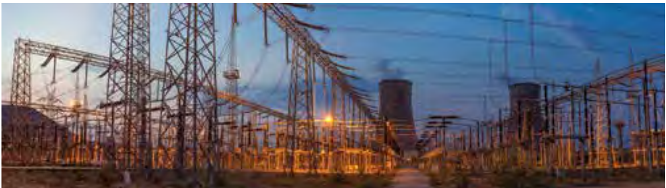
400 kV Switchyard commissioned by BHEL at Bellary Super Thermal Power Station, Karnataka
